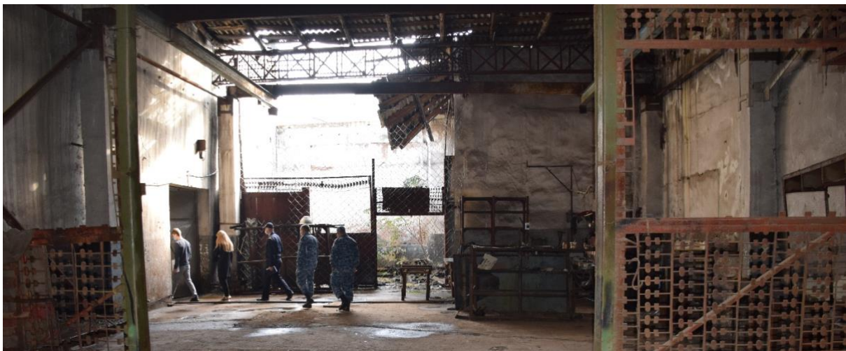
Picture 8 Workspace facilities are empty and in need of capital repairs, starting with the leaking roof
